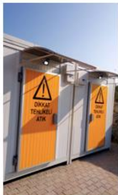
Refrigerated interim toxic waste storage
